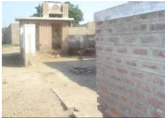
Broken Boundary Wall of School
