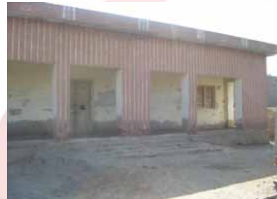
Broken Staircase of School
